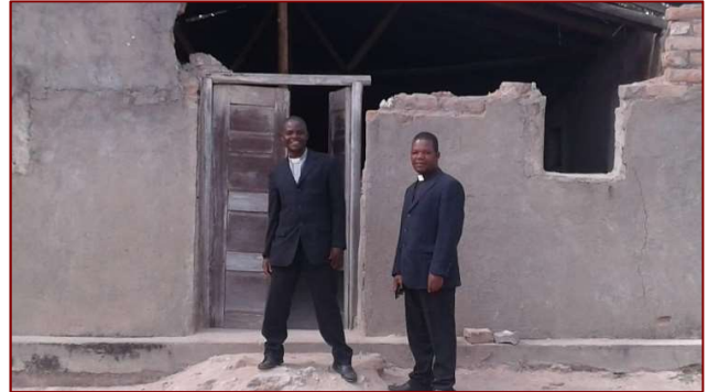
Pastors Samuel and Adolfo in front of the damaged Magodane prayer house
