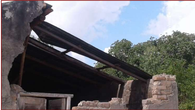
Damage to the Magodane prayer house
